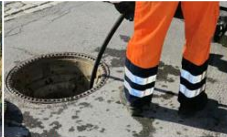
Sewer flooding (Anglian Water , Thames Water)
