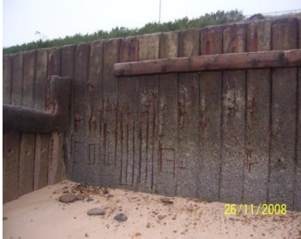
Hazlemere seawall before works commenced.
