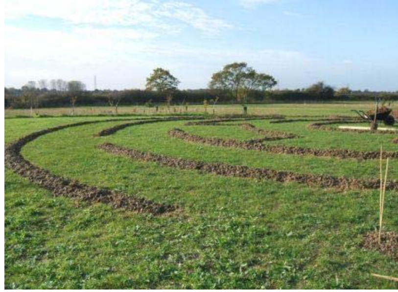
Stage 2: The outlined area after ground preparation by rotavating and weed killing.
