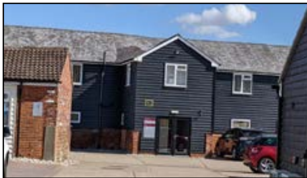
Figure 23 Loss of historic features within the barn complex can be seen with replacement windows, doors and roofing
