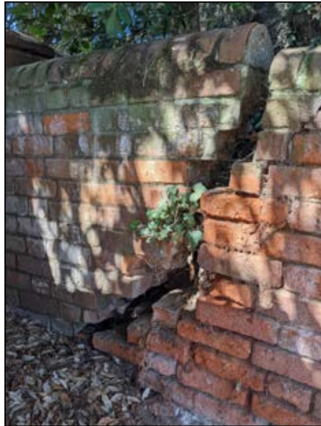
Figure 24 Damage to Brightlingsea Hall boundary wall
