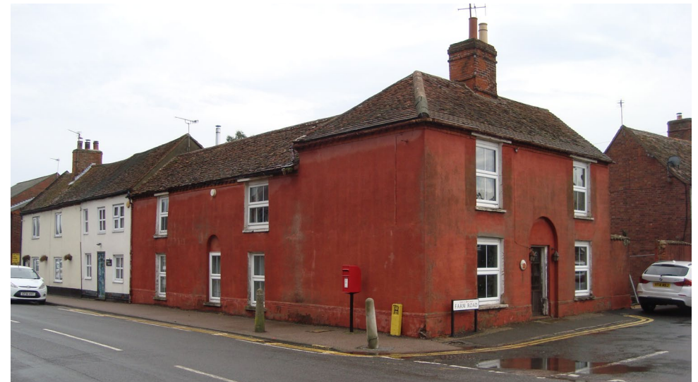
Figure 46 The insertion of inappropriate uPVC windows has harmed the historic and architectural interest of the Conservation Area
