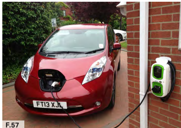
Figure 57: Examples of off-street mounted car charging points.
