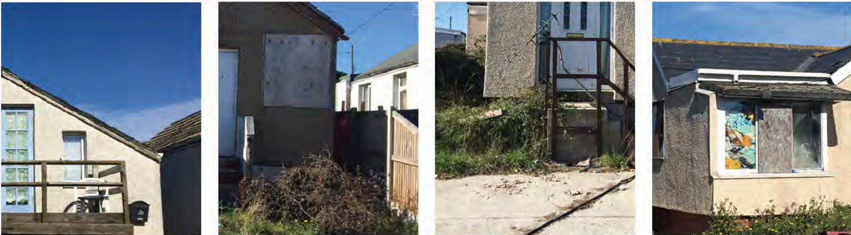
Fig. 49. Examples of occupied housing in poor condition.
