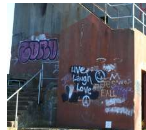
Figure 39 An example of vandalism at Beacon Hill Fort
