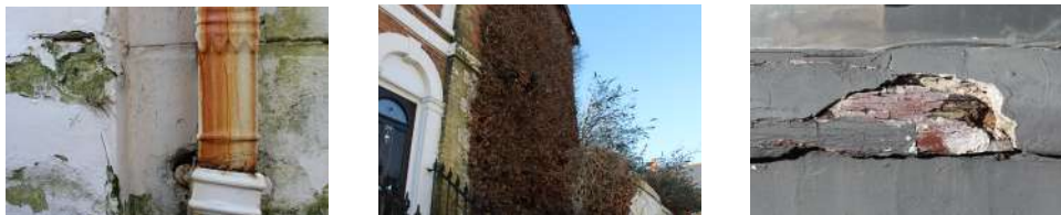
Figure 42 Examples of maintenance issues across the Conservation Area
