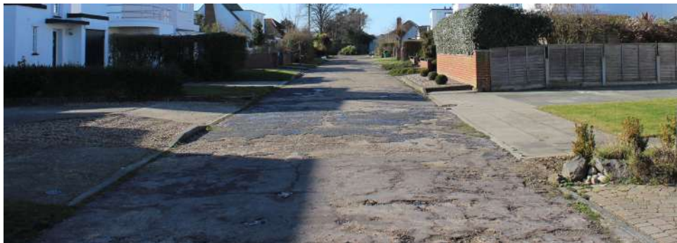
Figure 102 Uneven road surfacing
