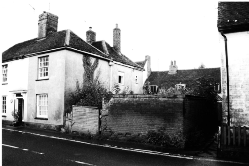
10. The side elevation to Oakwood and its garden adjoin alleyway between High Street and Queen Street. Both the building fabric and the garden boundary require urgent consideration.
