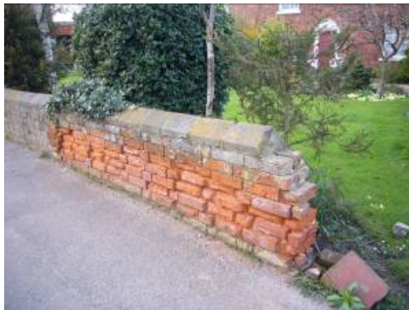
Boundary walls are a vulnerable element
