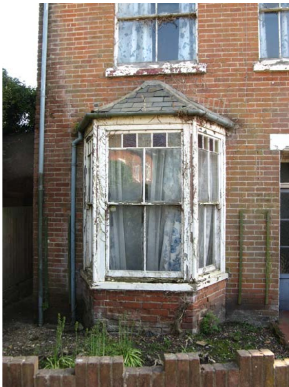
Clear evidence of decay that can lead to the loss of historical detail
