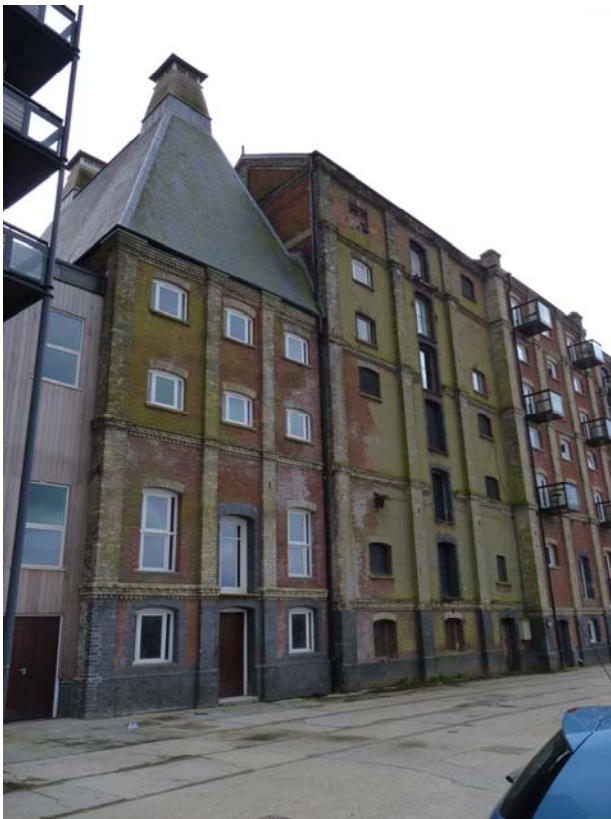
A Buildings-at-Risk Strategy would seek the reuse of the empty parts of the No.1 Maltings
