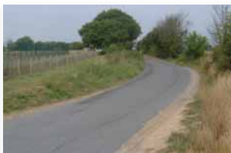
Verge damage in Pork Lane
