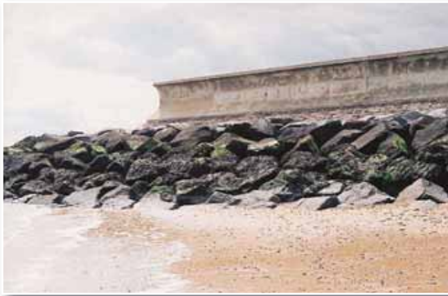
Weakened sea wall showing rocks employed for further protection
